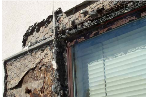
Figure 9 Damage at recessed window head resulting from lack of a soffit weep-drip screed
