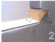
2 To slope the sill to the exterior, install a "sill wedge" and fasten it at each end. Next, cut the WRB at the jamb condition, about 2 1/2 inches above the sill, so that the upper edge of the WillFlash® CAPs can be "single-lapped" with the WRB.
