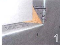
1 The wall has been covered with a weather resistive barrier (WRB), in this case a "housewrap," which is wrapped into the rough opening. Note the gaps at the sill-jamb condition.
