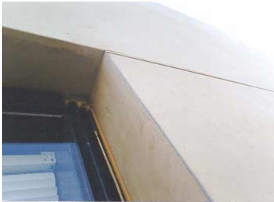
Deeply recessed window without weep at soffit suffered water penetration and damage at head
